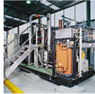
Figure 6: CFC, HCFC, HFC and halon destruction system
